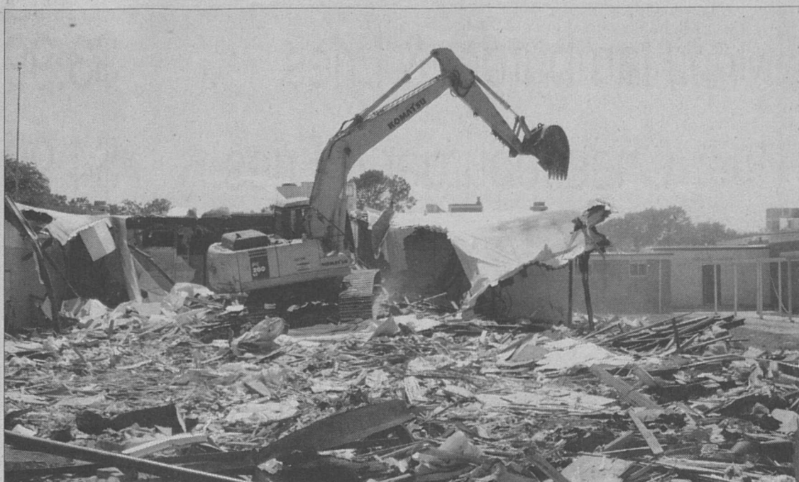
Demolition began Monday on Rice Consolidated's Tate Street Campus in Eagle Lake. Part of the facility is being torn down to make room for new construction. The remaining facility will be remodeled. When complete sometime next spring, the facility will house fourth, fifth and sixth grade students and will be called the Eagle Lake Intermediate School. The project will cost about $2.7 million dollars and includes some work in Altair as well.
